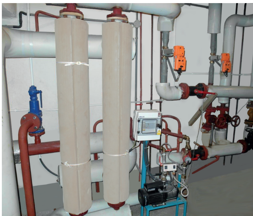
One of the heating stations equipped with globe valve actuators from Belimo
