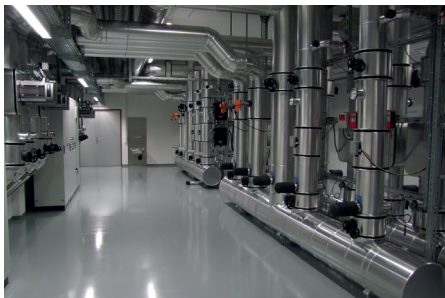
Heating/cooling control centre
