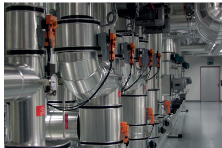
Heating/cooling control centre
