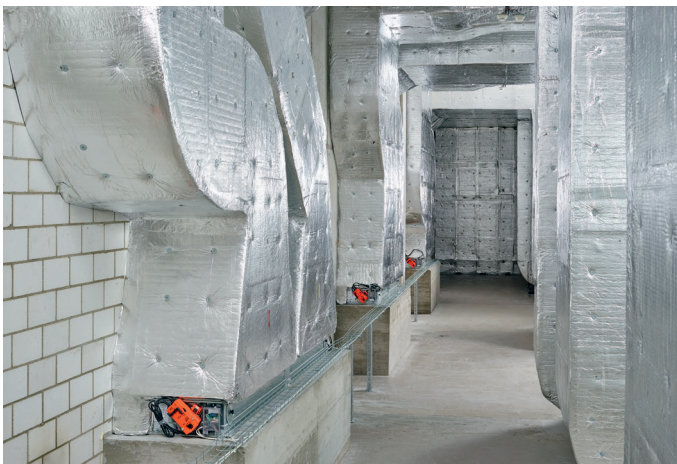
Once the air handling unit is switched off, the fire dampers close automatically, thus securing the fire compartments to the tenants' premises.
