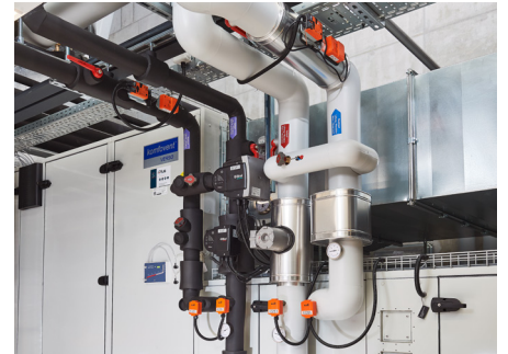
Circuits for heating/cooling coils of ventilation with electronic pressure-independent valves (EPIV) and temperature sensors.
