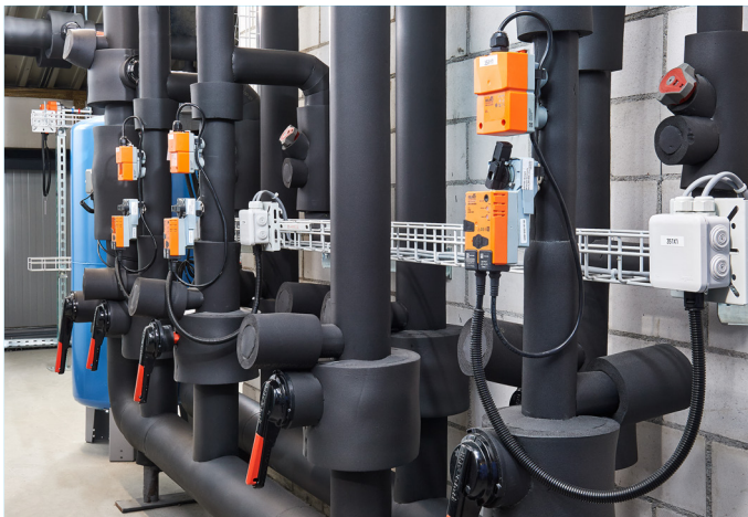
Cooling distribution with electronic pressure-independent valves (EPIV).
