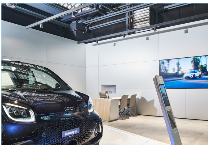
Optimum room climate in the showroom with the help of fan coils
