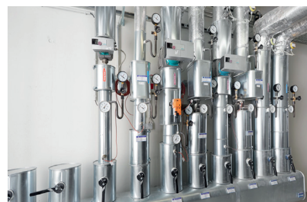
The heating station with three connected circuits for ventilation, offices and heat supply in the technical centre.
