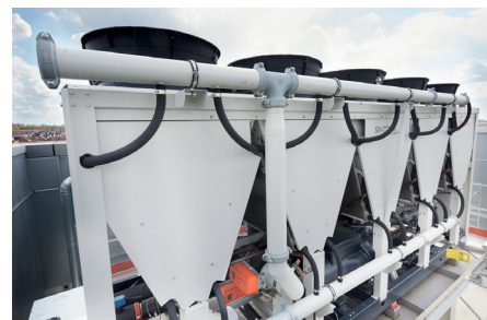
Cooling for ventilation and air conditioning systems.
