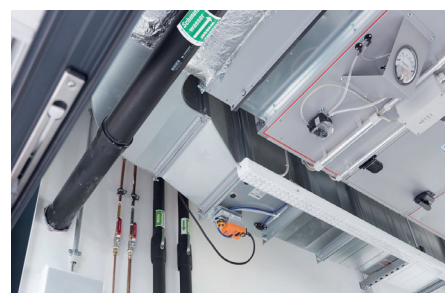
Volumetric flow controllers ensure constant conditions for air and room climate in the laboratories.
