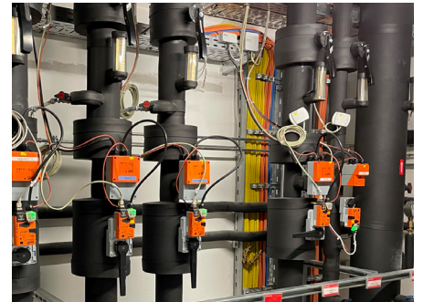
The Belimo Energy Valves dynamically control and monitor all hydronic manifold circuits by continuously measuring flow rates and water temperatures.
