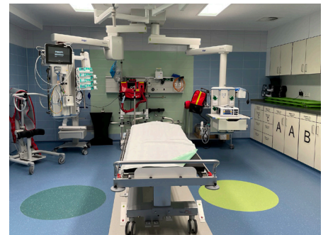
Intelligent and efficient HVAC systems ensure that all rooms in the Ludmillerstift Hospital are heated, cooled and ventilated as required.
