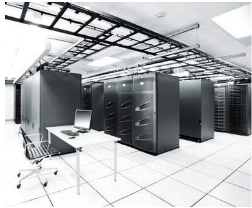
Abb. 109: Typical CRAC devices.
