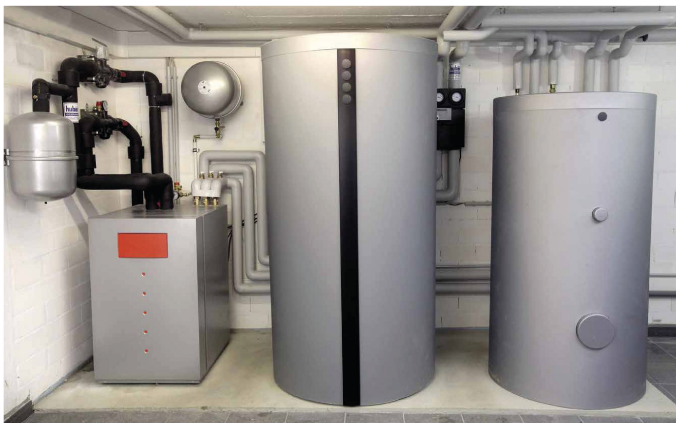
Abb. 114: Heat pump with potable hot water storage tank.
