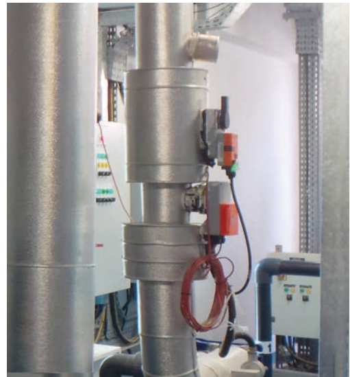
Abb. 82: The supply of the fan coils is equipped with the Belimo Energy Valve™.
