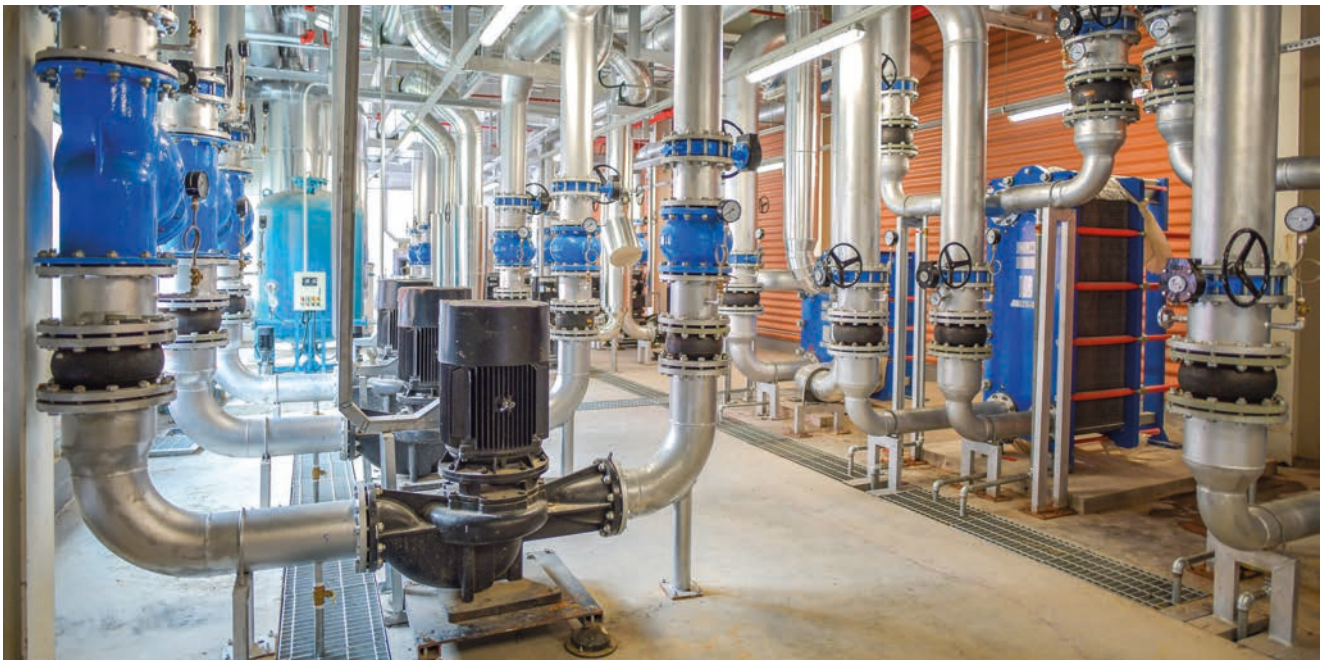
Abb. 60: Heat exchange station
