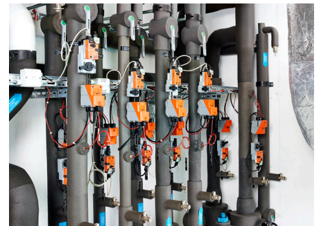
Belimo energy valves of the third generation have been in use at NEST since 2016.
