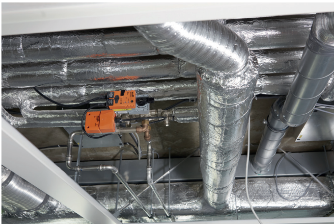
The electronic pressure-independent 6-way EPIV zone valves installed in the ceiling control the flow of hot and cold water.
