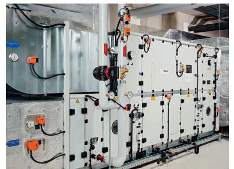
Air handling unit equipped with sensors, damper actuators and electronic pressure-independent characterised control valve EPIV from Belimo.
