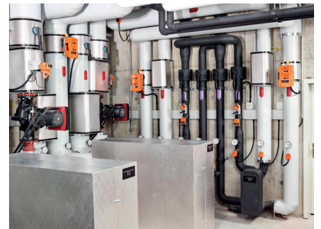
Tight-closing Belimo open/close butterfly valves in the cooling and heating station.
