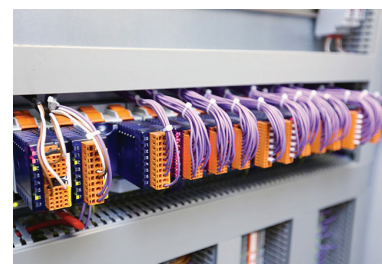
New BMS head end in the technical control centre for the cold/hot water supply
